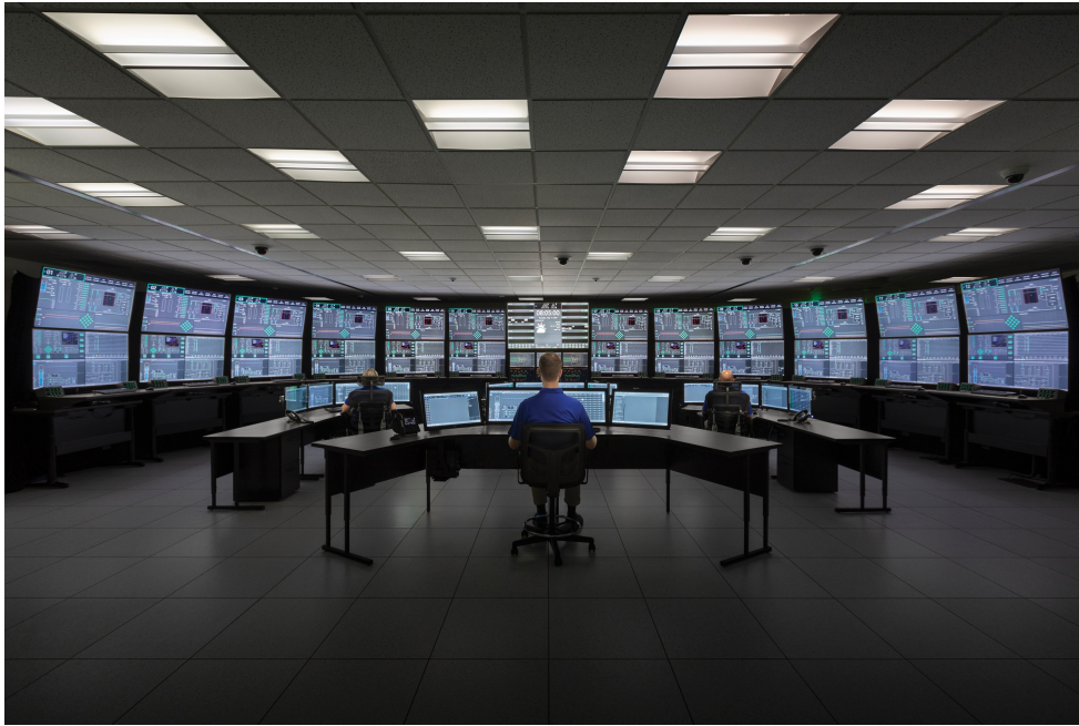
NuScale Control Room Simulator
