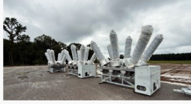
Delivery of Entergy 230 kV breakers
